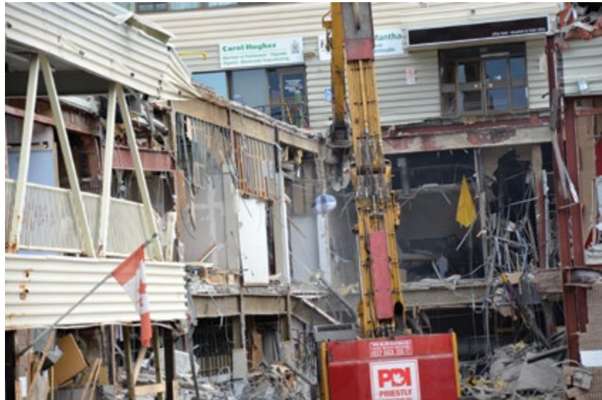
Figure 2.6.10 Mr. Priestly at work removing debris from the collapsed zone in the Mall
