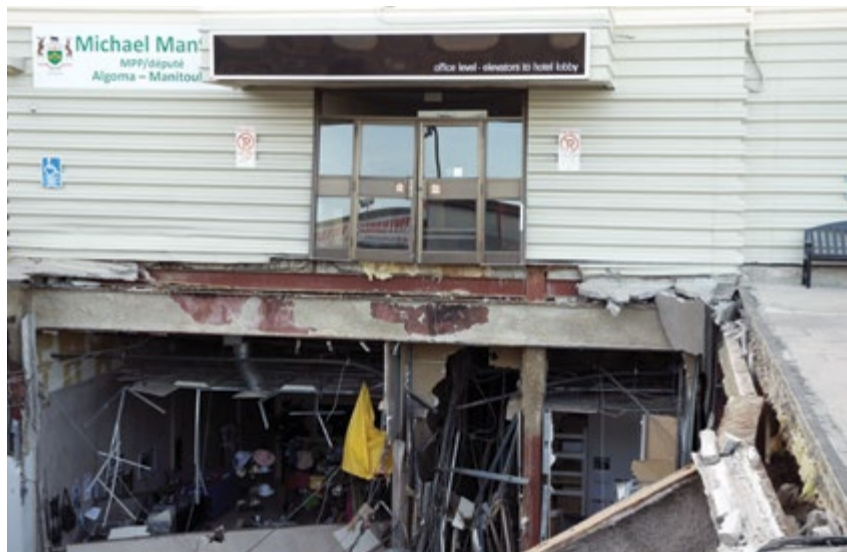
Figure 2.6.11 The corner where some small pieces of concrete may have fallen during the clearing of the Mall
