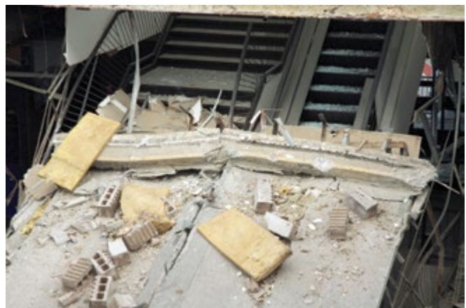
Figure 2.4.2 Debris on escalator
