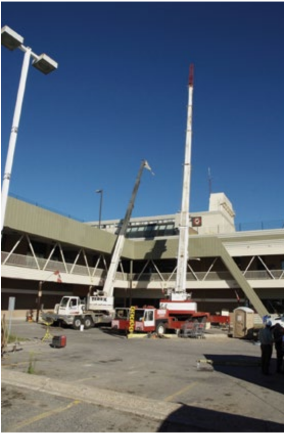
Figure 2.4.6 The red part of the larger crane is the jib and the boom is white
