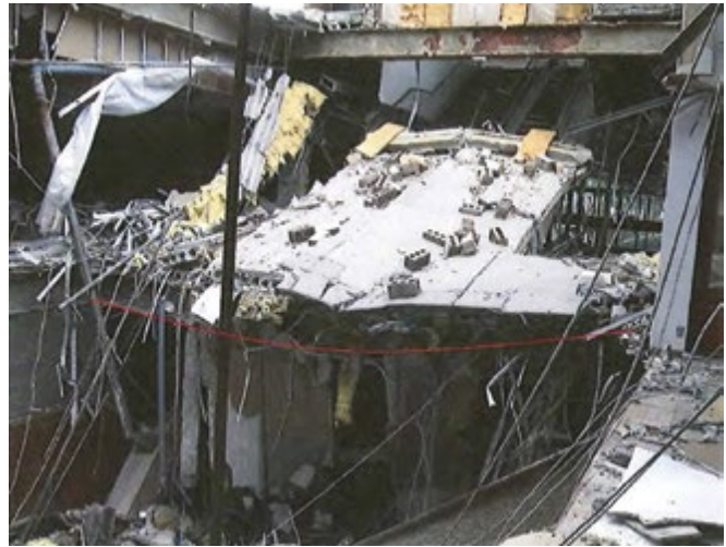
Figure 2.4.1 Bow in beam under the escalator
