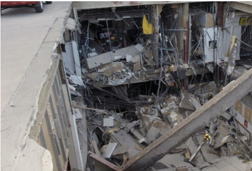
Figure 2.3.1 The collapse zone
