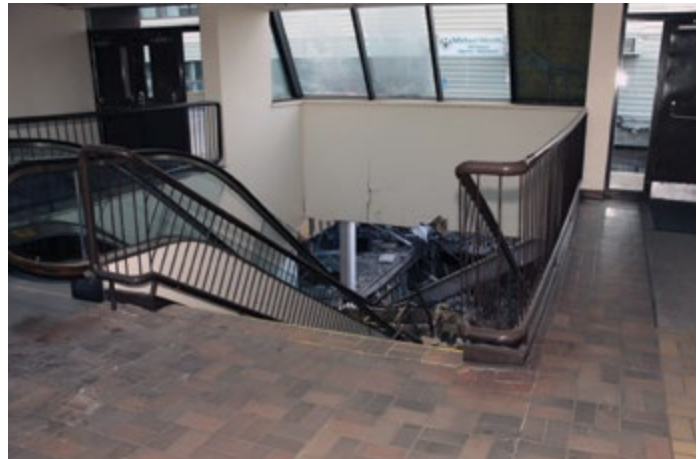
Figure 2.3.2 Staircase with debris: looking into the collapse area
