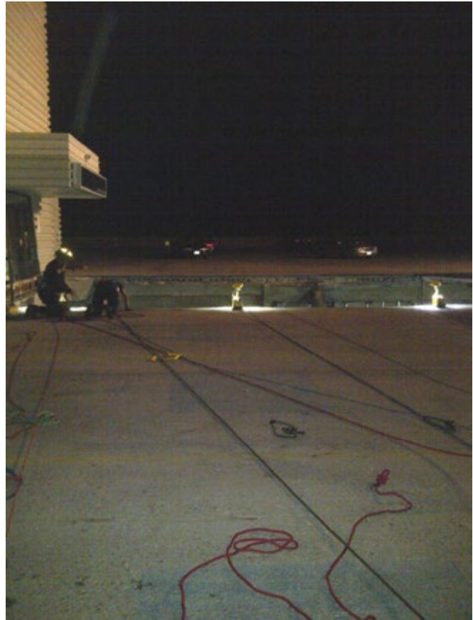
Figure 2.3.8 UCRT members set up portable lighting on the roof of the Mall
