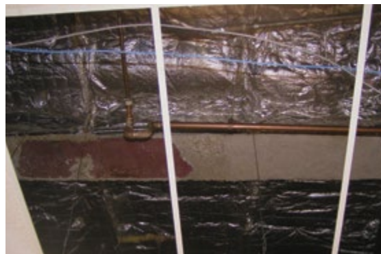
Figure 1.10.4 Rust and missing fireproofing caused by water leakage on the I-beam above the Bargain Store
