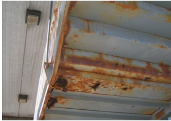
Figure 1.10.7 The rusted steel stairway outside the Mall and in front of the Foodland store
