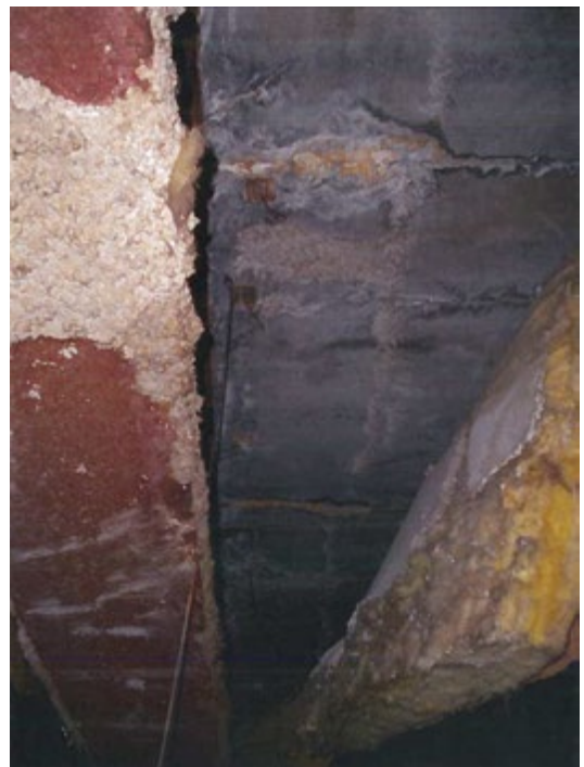
Figure 1.10.8 Rust and missing fireproofing on the beam at gridline 16 – the one that later collapsed
