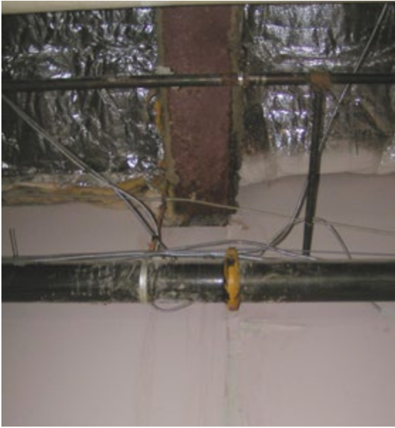
Figure 1.10.5 Rust and missing fireproofing on the bottom of the structural steel and smaller pipe in the service hall behind the Dollarama store
