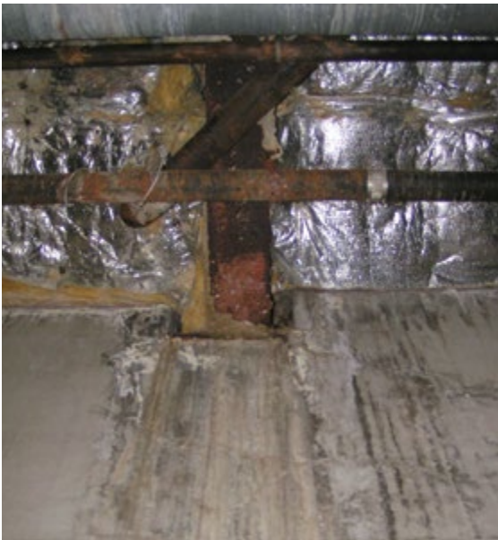
Figure 1.10.6 Evidence of water leakage, missing fire proofing, and rust on the structural steel in the service corridor behind the Library
