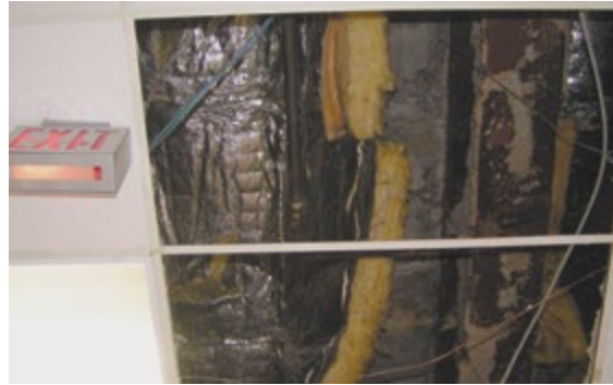
Figure 1.10.2 Missing fireproofing and rust on a structural steel beam in the upper level of the Mall above the lottery kiosk
