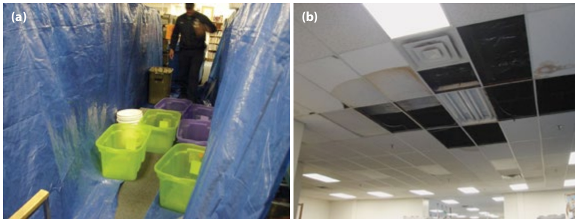
Figure 1.5.3 (a) Buckets and tarps are used to catch leaks and cover large sections of books in the Library; (b) numerous tiles missing in the Library ceiling due to leaks
