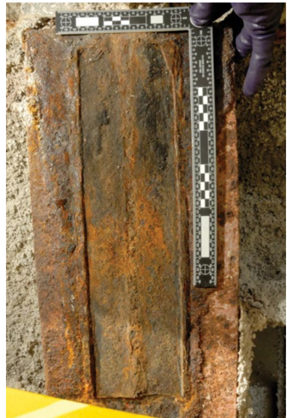
Figure 1.3.7 Face of the column flange at gridline G-16 and the beam and angle that were connected to the column flange before failure
