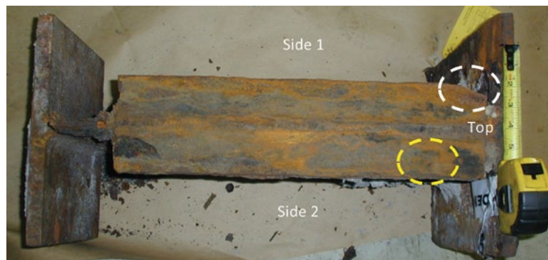
Figure 1.3.6b Top view of the failed beam connection showing that the angle and bolted connection were severely corroded
