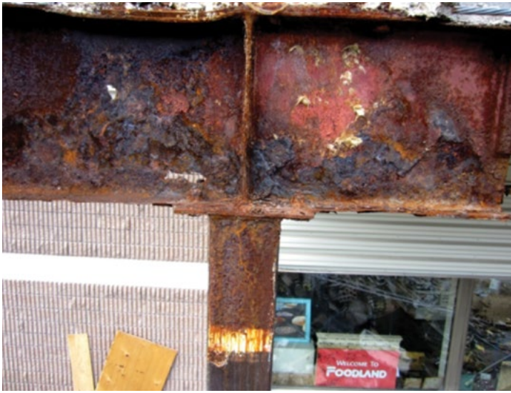
Figure 1.3.5 Severely corroded connection at the pedestrian walkway located at gridline E-13x
