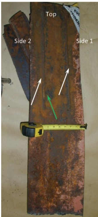
Figure 1.3.6a Column flange of failed connection
